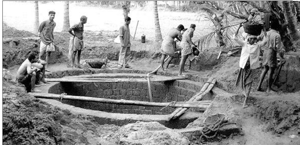
Source construction in progress – open well being constructed by the Theru BG in Pilicode GP – the construction is done through community contracting method, avoiding contractors.
