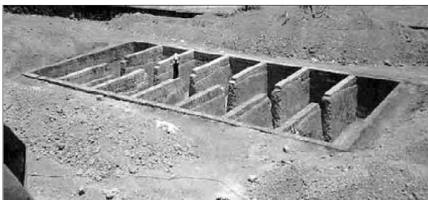
The 4.25 lakh litre capacity underground storage tank being constructed in the campus of the District Panchayat office in Kasaragod for the model roof top rain water harvesting scheme.
