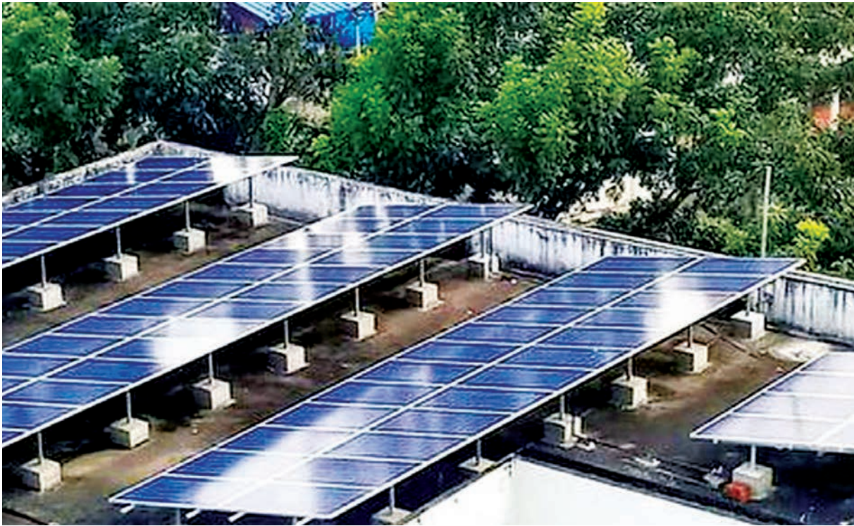
KSEB Solar Projects
