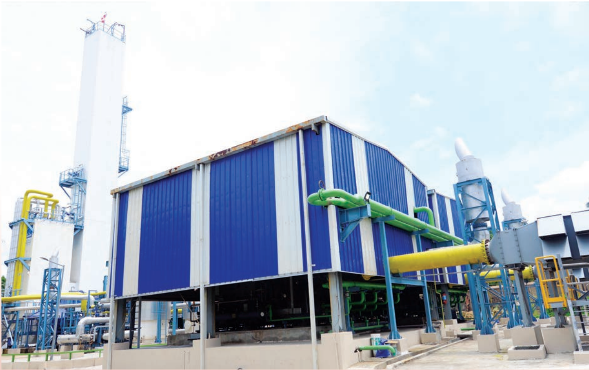
Oxygen plant at KMML, Chavara
